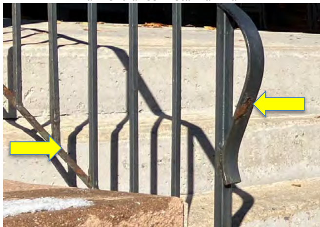
Main entrance metal handrail corrosion
