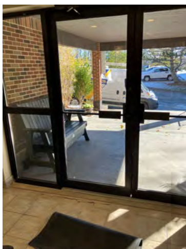
Cracked entrance foyer tiles
