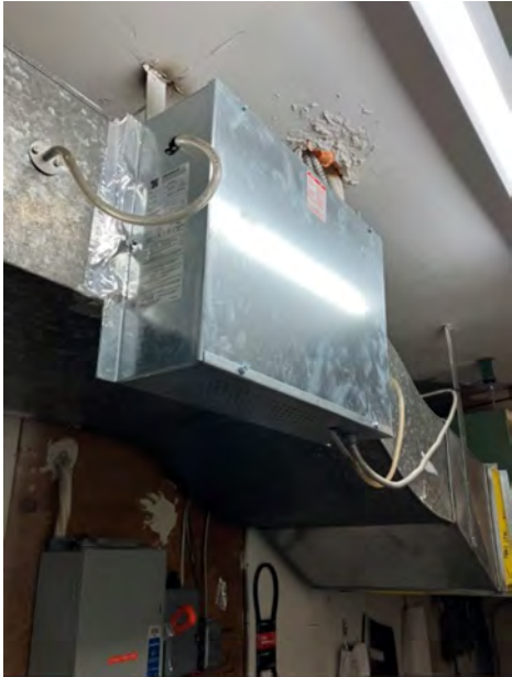
Electric duct heater replaced in 2023
