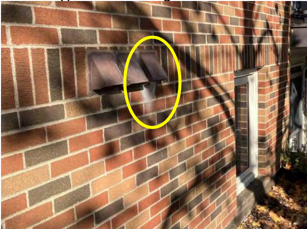
Dryer lint buildup in exhaust duct hood
