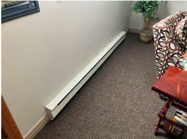
Common room electric baseboard heater
