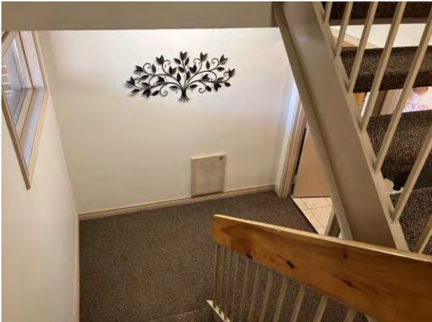
South stairwell electric wall unit heater
