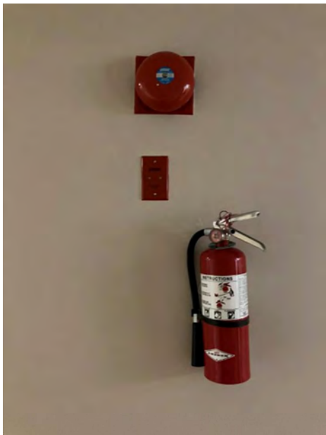
Corridor fire protection equipment
