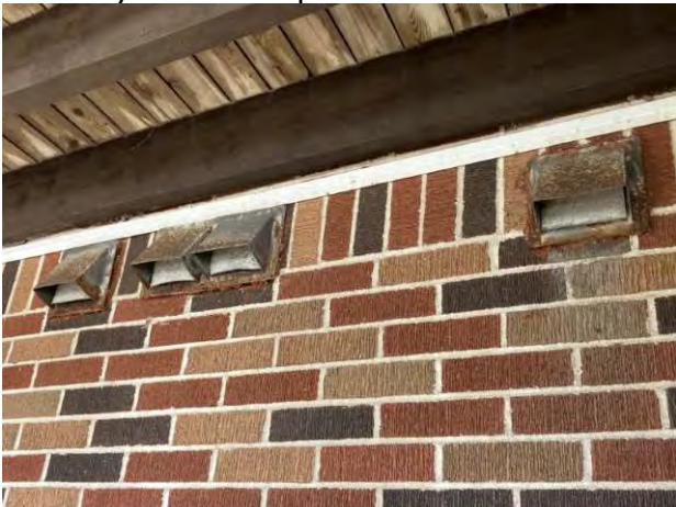
North elevation corroded and poorly sealed exhaust duct hoods
