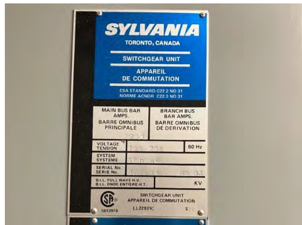
1200 amp fusible disconnect nameplate
