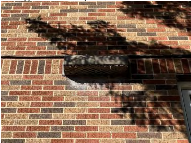
Dryer lint buildup in exhaust duct hood with pest guard screen
