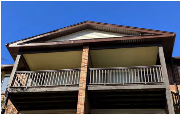
Defects in east elevation fascia above balconies
