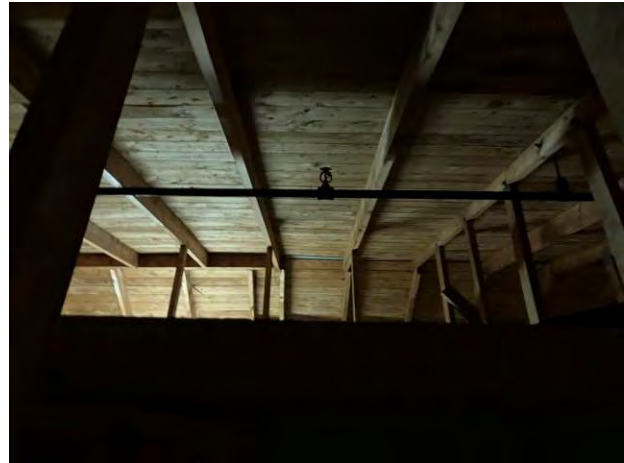
Fire safety system sprinkler head in attic
