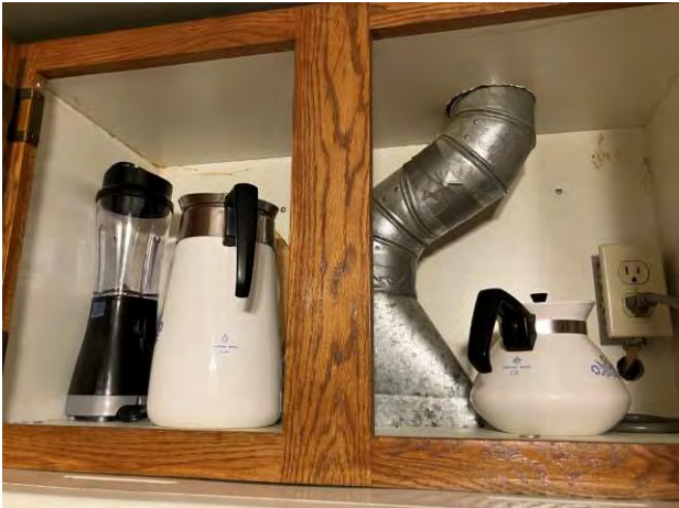
Typical kitchen range exhaust duct
