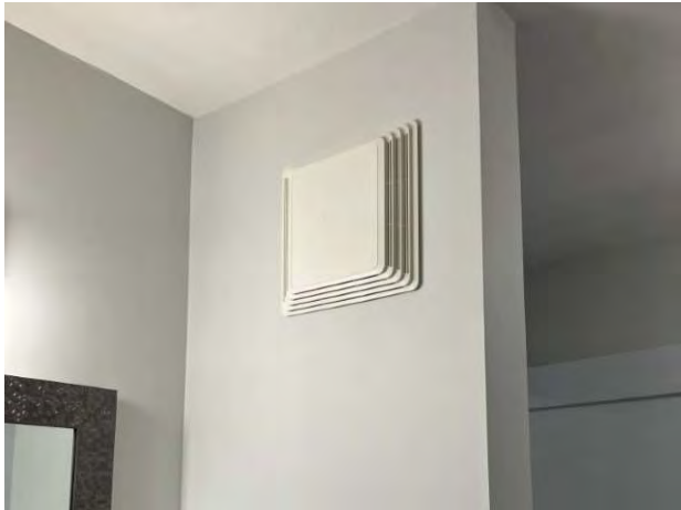
Typical bathroom exhaust fan
