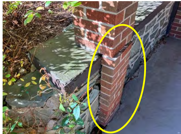
Main entrance brickwork in need of repair
