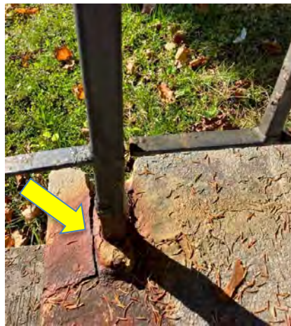
North entrance landing cracks
