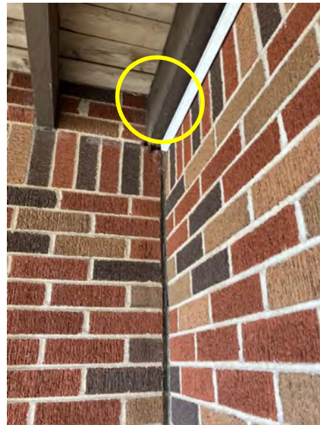
Void in brickwork in mechanical room exterior entrance vestibule
