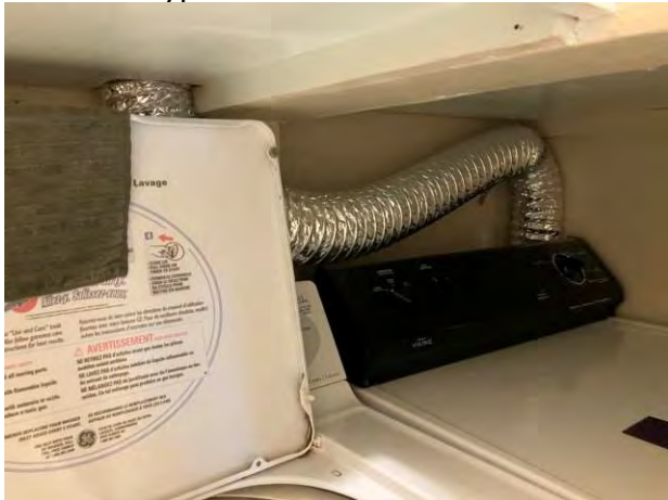
Typical clothes dryer flexible exhaust duct
