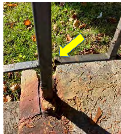
North entrance metal handrail corrosion
