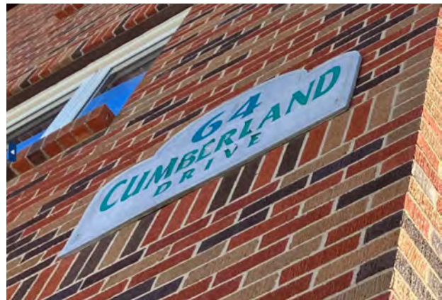
View of existing building unit sign showing signs of wear
