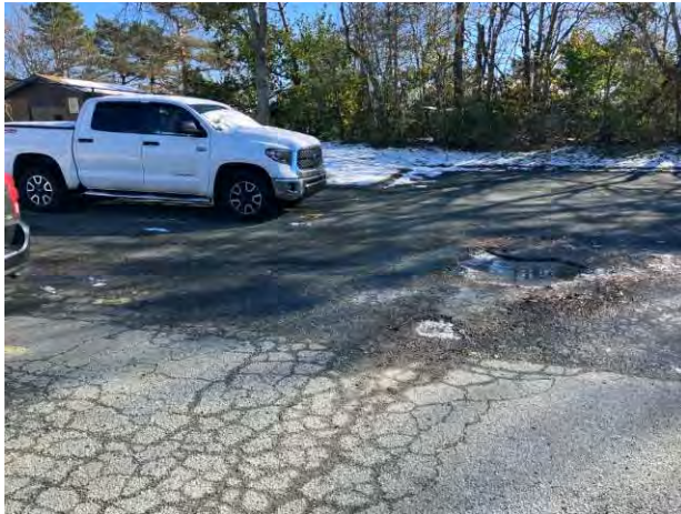
Asphalt parking lot on northeast side of property, with damaged section
