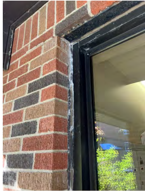
Caulking between main entrance metal door frame and brick veneer showing signs of wear
