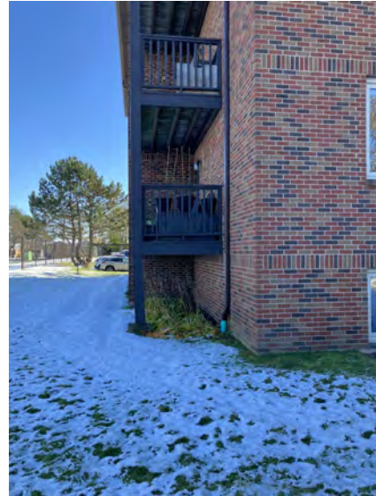
North balcony timber post out of plumb
