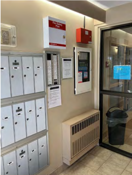
Main entrance vestibule electric wall unit heater
