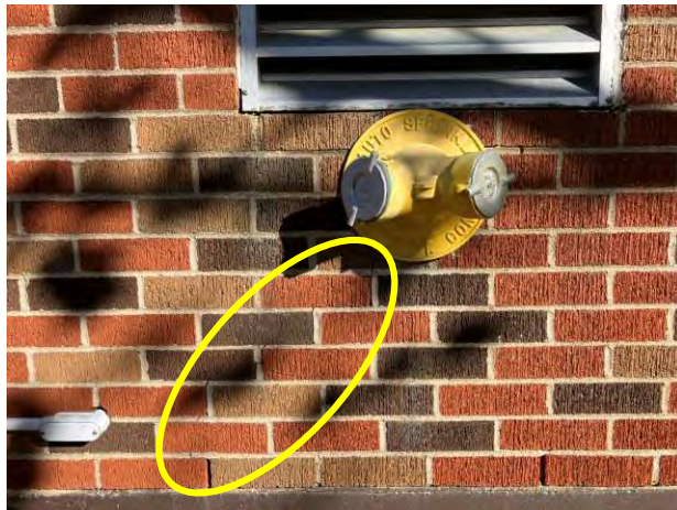
Cracked mortar beneath fire department connection on south elevation
