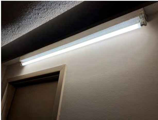
Typical LED corridor lighting
